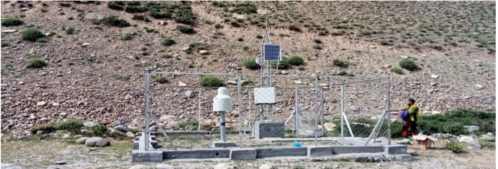
RTDAS ARG SITE FOR DATA COLLECTION
