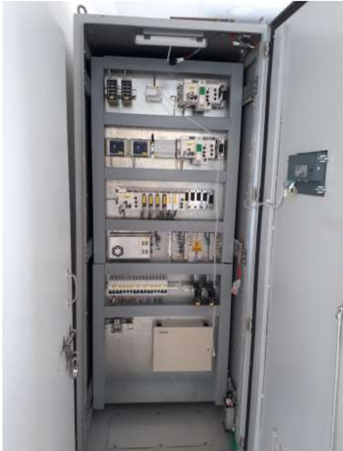
MAIN PLC PANEL
