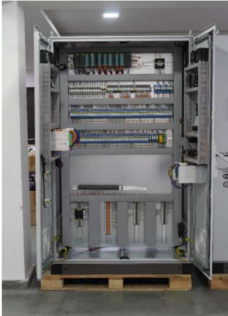
HOT REDUNDANT MAIN PLC PANEL
