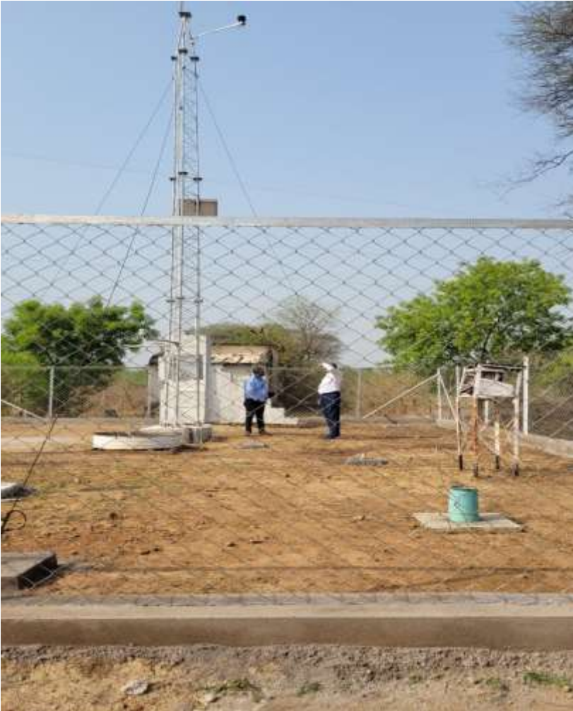
WEATHER STATION WITH TRIPOT AND FENCING
