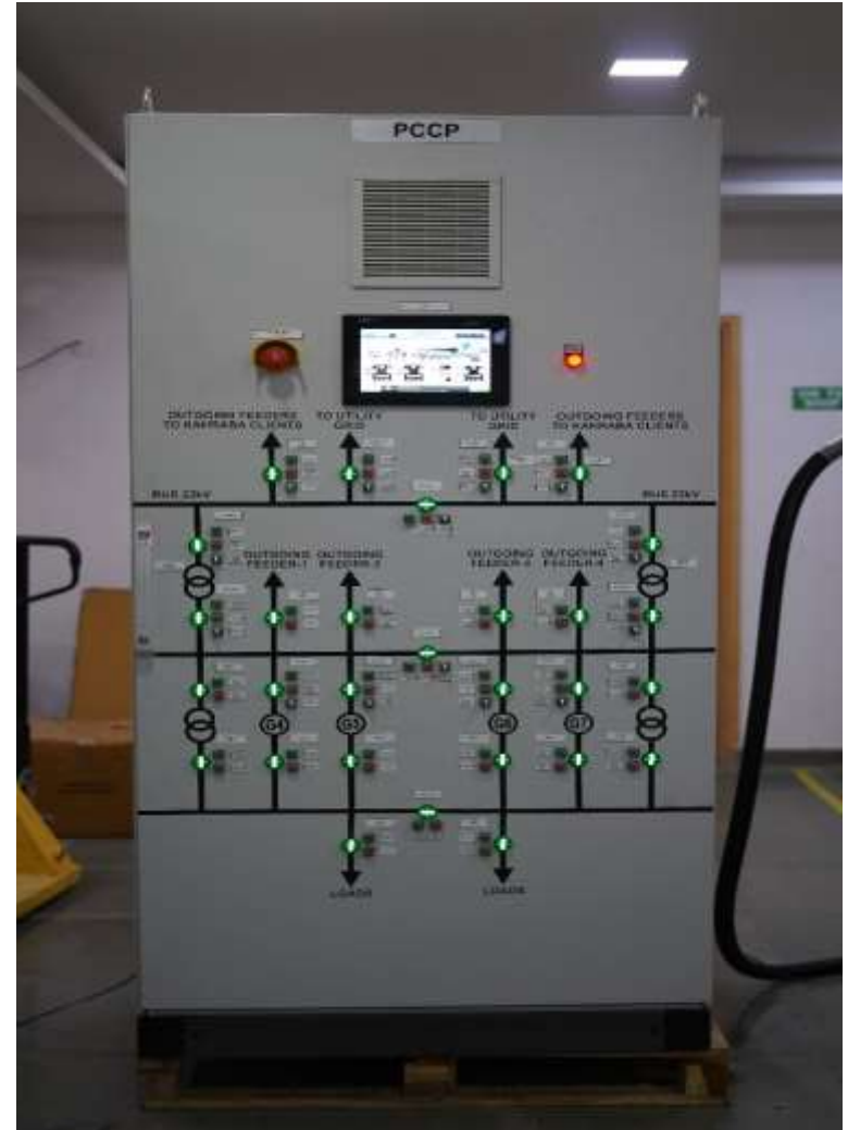
INDUSTRIAL PLC WITH HMI PANEL
