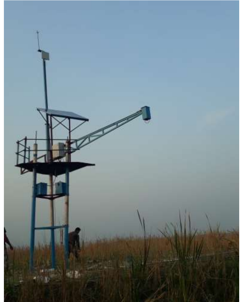
FLOOD ALARM SYSTEM WITH RF COMMUNICATION SYSTEM
